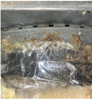
Duct Sealing Before
