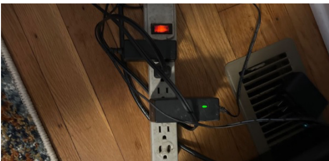
Existing Power Strip
