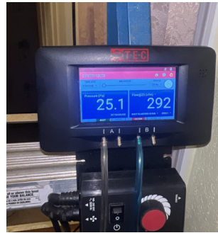
Duct Sealing Reading Before
