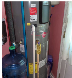
New Heat-Pump Water Heater
