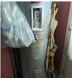
Existing Water Heater
