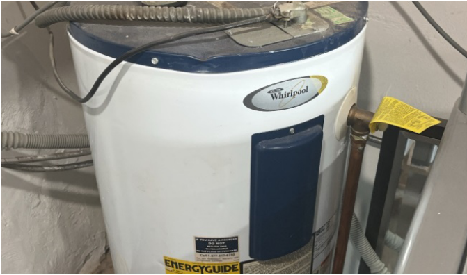
Existing Water Heater Before Wrap
