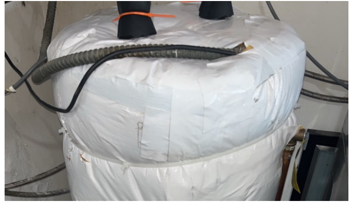
Water Heater with Wrap
