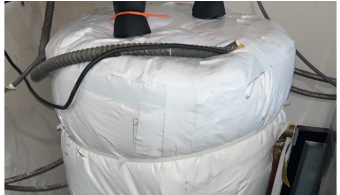
Water Heater with Wrap
