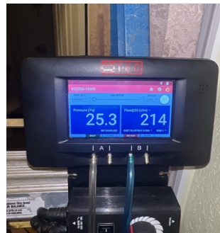
Duct Sealing Reading After
