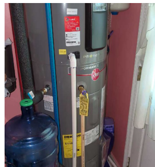
New Heat-Pump Water Heater
