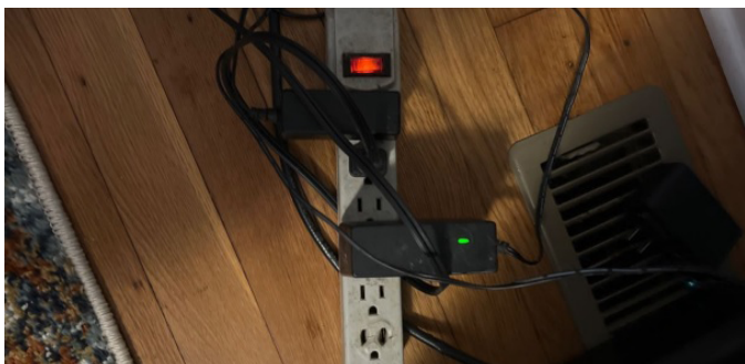
Existing Power Strip
