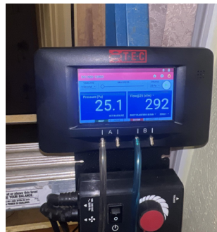
Duct Sealing Reading Before
