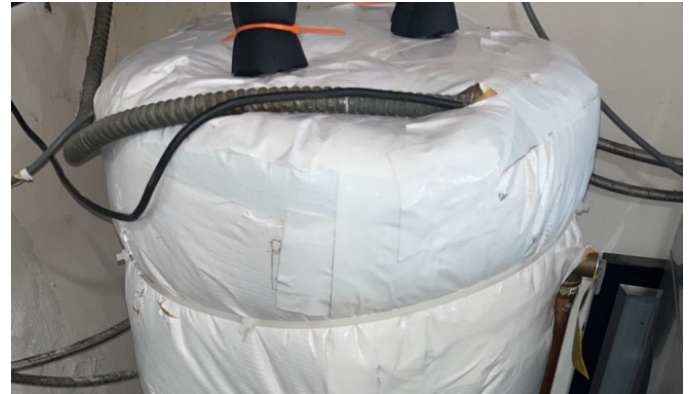
Water Heater with Wrap
