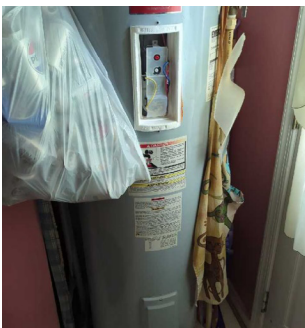
Existing Water Heater
