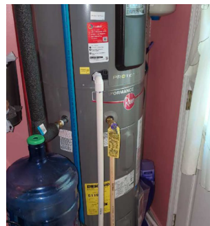
New Heat-Pump Water Heater
