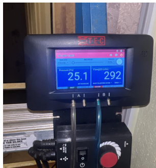
Duct Sealing Reading Before
