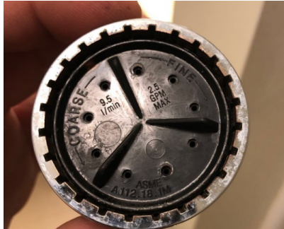
Existing Showerhead GPM
