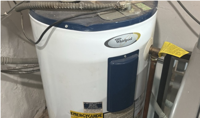
Existing Water Heater Before Wrap
