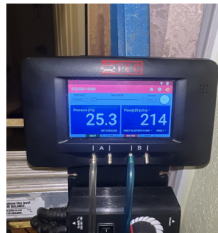
Duct Sealing Reading After
